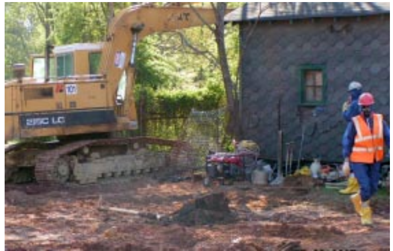
Contractors connect new sanitary lines to the South Bound Brook municipal system.
