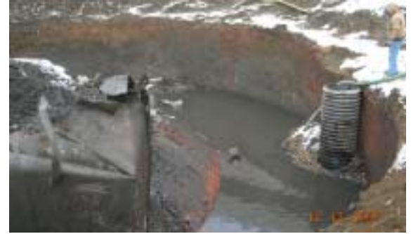
Contaminated soil was excavated from one of the 1800s brick gas holders during site remediation.
