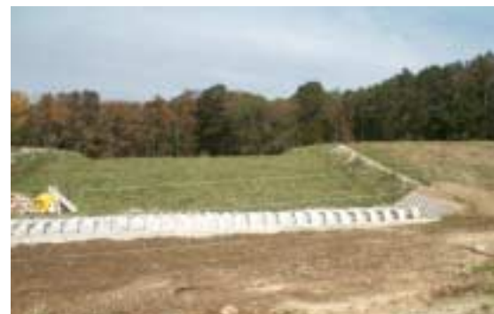
Overall photo of the larger downstream pond (top) and its Emergency Spillway and Stilling Basin at the larger downstream pond.
