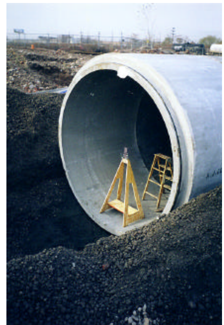
The 10-foot diameter pipe was designed to accommodate loads from fill and parking areas constructed over the pipe.
